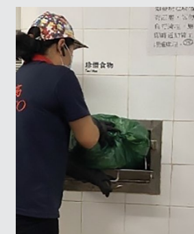
Refuse chute inlets
