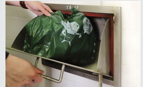
Inlet of refuse chute on individual floor
