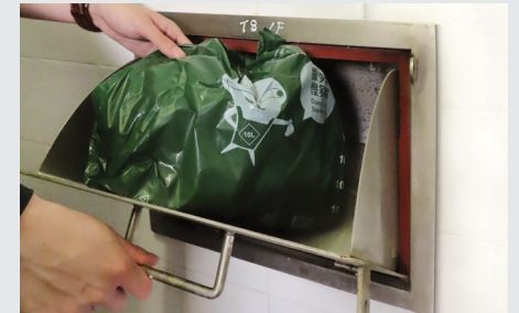
Inlet of refuse chute on individual floor
