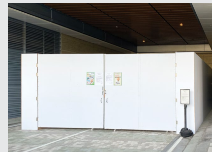
Oversized waste reception areas (i)
