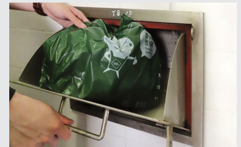
Inlet of refuse chute on individual floor
