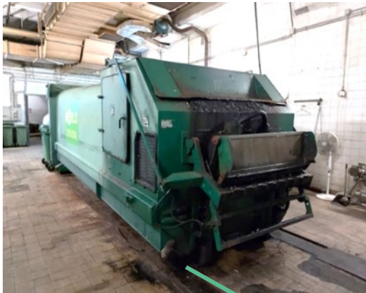
1. Mobile Refuse Compaction System (Refuse Compactor)
