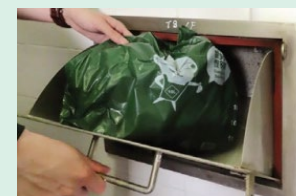
Inlet of the refuse chute on individual floor
