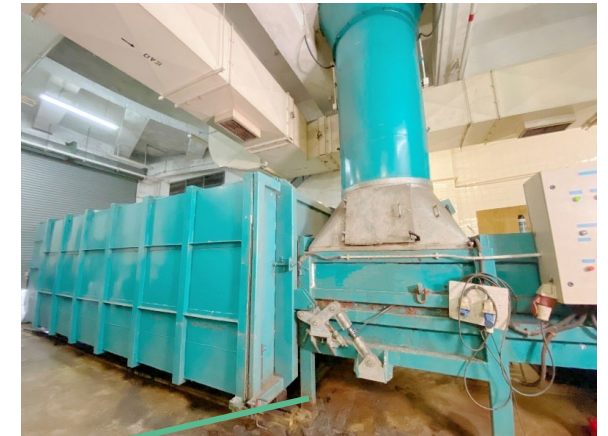
3. Automatic Refuse Collection System
