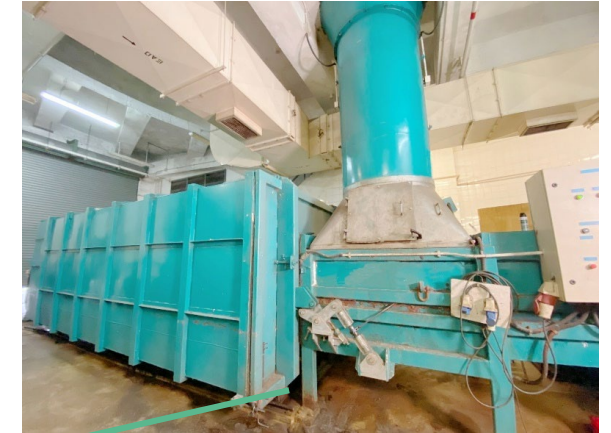
3. Automatic Refuse Collection System
