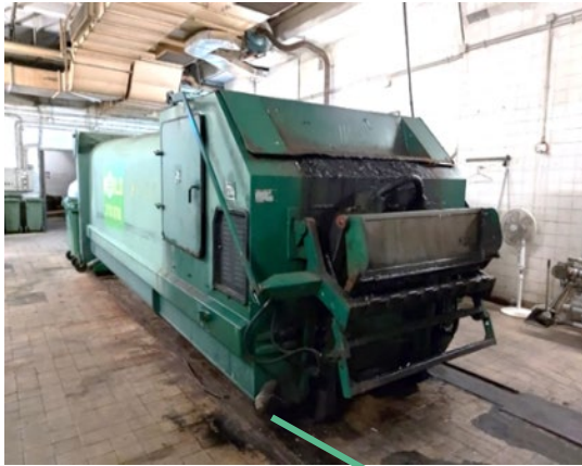
1. Mobile Refuse Compaction System (Refuse Compactor)
