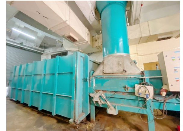
3. Automatic Refuse Collection System
