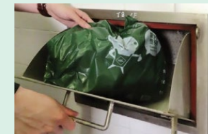
Inlet of the refuse chute on individual floor
