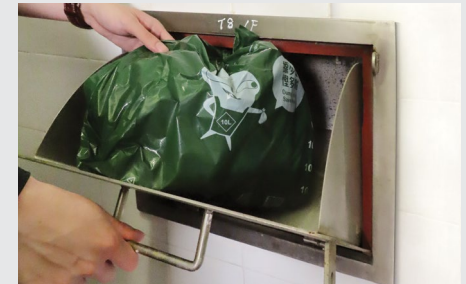
Inlet of refuse chute on individual floor
