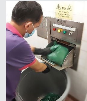
Refuse chute inlets that are linked to ARCSSs
