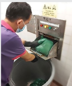
Cleansing workers deposit waste properly wrapped in designated bags into inlets that are linked to ARCSs
