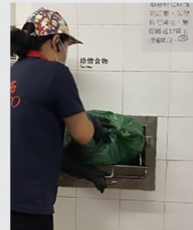
Refuse chute inlets
