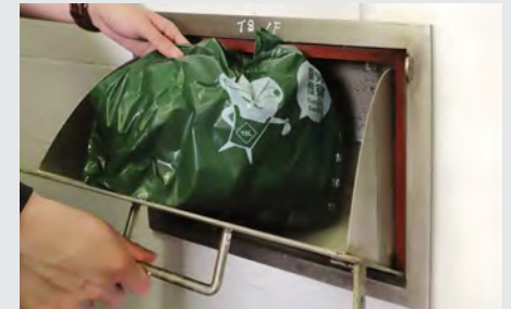
Inlet of refuse chute on individual floor
