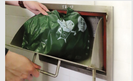
Inlet of refuse chute on individual floor
